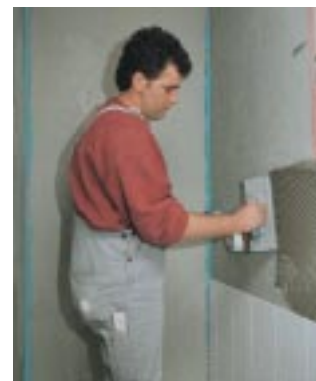
6. After the waterproofing PCI Lastogum is dry tiles and flags can be laid with PCI-Tilefast 6.
