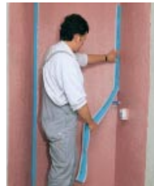
3. Fix the PCI-waterproofing tape 120 with PCI-Lastogum (red) in corner joints and floor/wall junctions.
