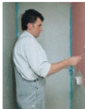
5. After an evaporation time of 2-3 hours apply the second protective coating with PCI-Lastogum (grey). The first coat of PCI-Lastogum (red) must not be visible.
